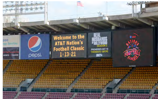
Installed state-of-the-art LCD flat panel digital signage system.
